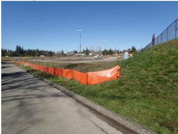
Silt fence at south side of parking area NE
